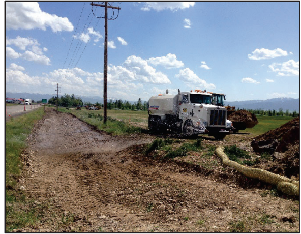
Figure 113. Sprinkling water for dust control on a pathway construction project, Driggs, Idaho.
